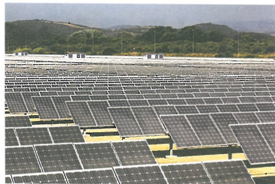
A field of solar panels
